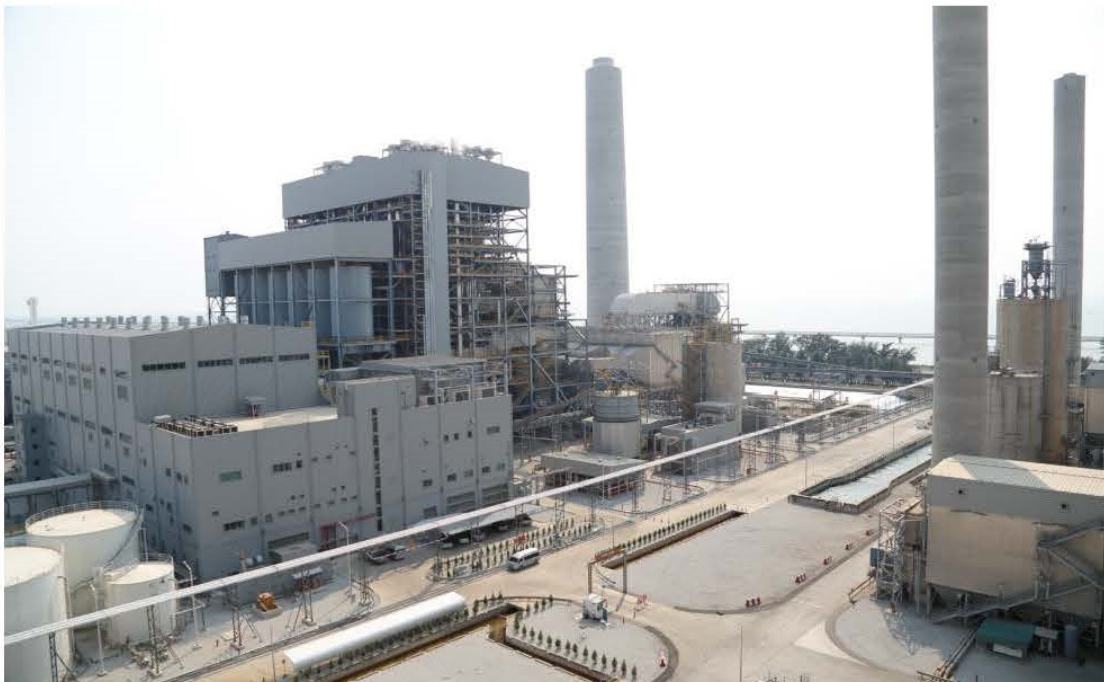
Gheco-One 660 MWe power plant in Rayong Thailand, owned by Glow Energy part of ENGIE
